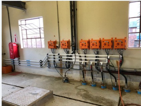
LOCAL MOTOR CONTROLS AND SERVICE PIPEWORK
