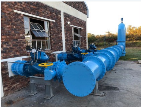
EXTERNAL VALVE AND PIPEWORK MANIFOLD
