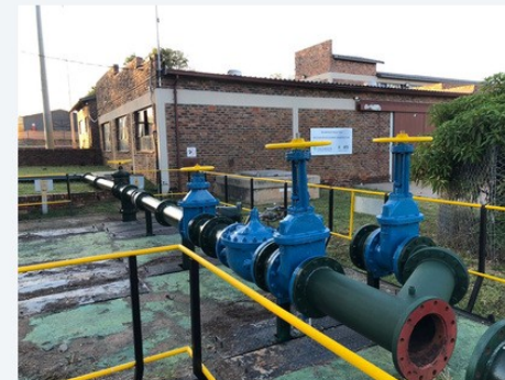
ISOLATION VALVES AND ABOVE-GROUND PIPELINE
