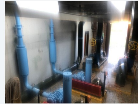
PUMP ROOM AND VERTICAL PIPEWORK
