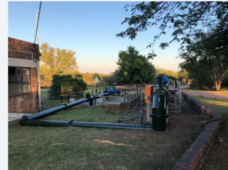
EXTERNAL PIPELINE AND TREATMENT INFRASTRUCTURE
