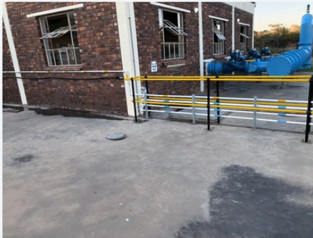
EXTERNAL PIPEWORK AND SAFETY HANDRAILS
