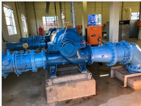
PUMP, COUPLING AND PROCESS PIPEWORK
