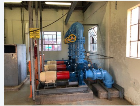
MULTI-PUMP STATION AND MOTOR DRIVES
